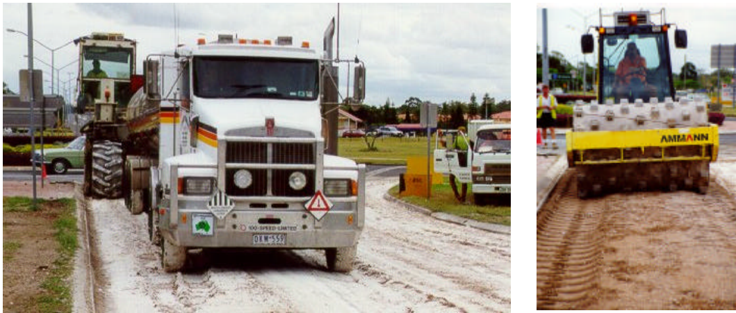
Figure 4 – Foamed bitumen mixing using the road recycler with foaming apparatus (left) and initial compaction using a pad foot roller (right).
